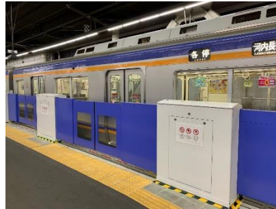
Large-opening platform gates installed at Namba Station
