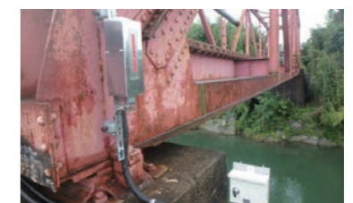
Bridge Abnormality Detection System (Kinokawa River bridge on the Koya Line)
