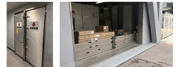
Watertight door (left) and a tide embankment (right) (Tamade General Office)
