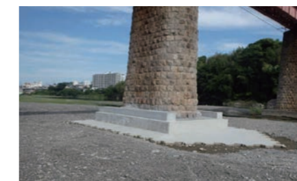
Construction to prevent scouring on the P3 bridge pier at the Kinokawa River Bridge on the Koya Line
