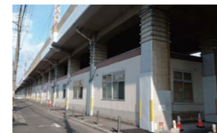
Seismic reinforcement of elevated bridge columns between Kohama Station and Sumiyoshitaisha Station
